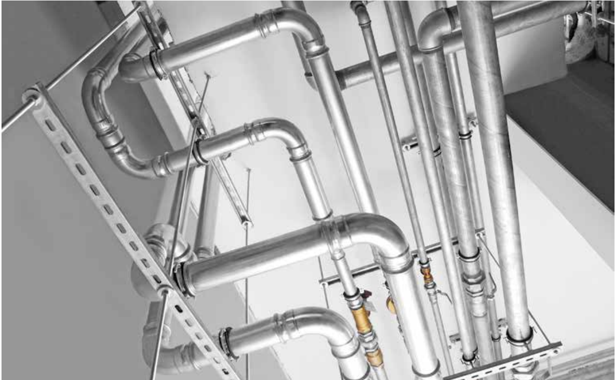
Exemplary KAN-therm Inox installation
